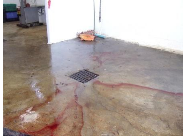
Figure 7A: Drainage in collection centre
