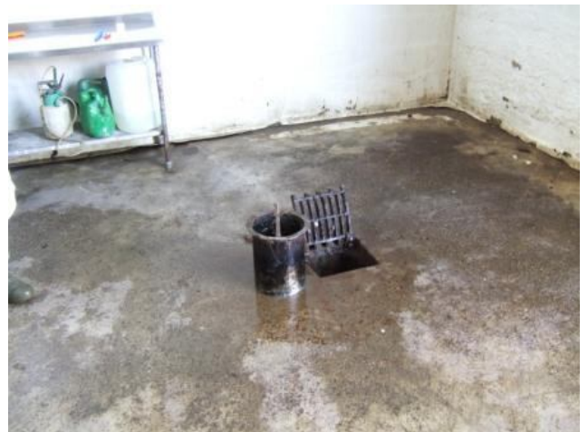
Figure 8A: Trap with 6mm holes that is suspended below drain
