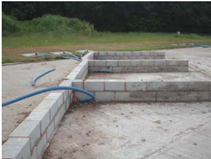
Empty bays showing drainage system and underground drainage tanks in the background.
