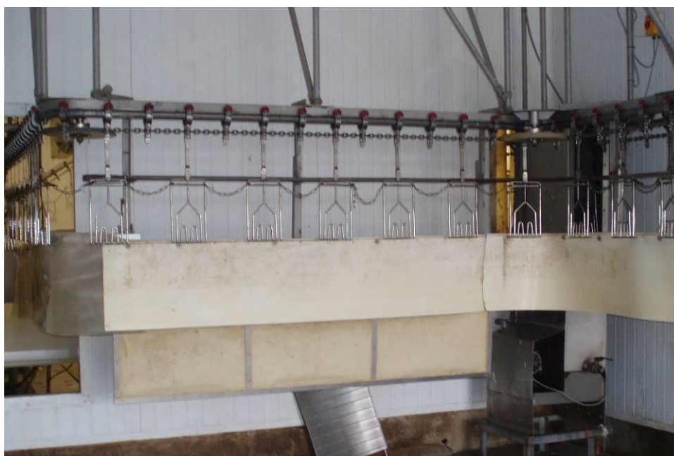
Figure 3 Conventional shackle line and breast rub strip in the plant before conveyor installation. (Note – shackle spacing was halved prior to all trial work for unrelated operational reasons – see Figure 4)
